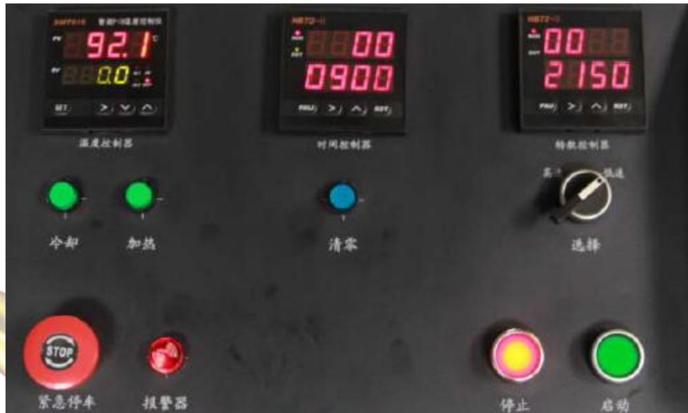
Fig.3 Electric cabinet and control panel
