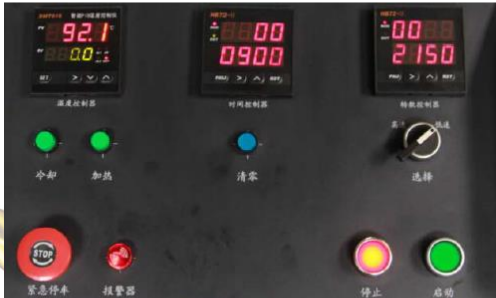
Fig.3 Electric cabinet and control panel
